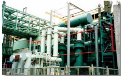
Thermal Power Generation Transformer 345kV-330MVA
