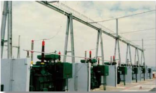
Power Transformer 345kV-500MVA
