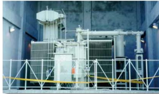
Cogeneration Transformer 161kV-150MVA
