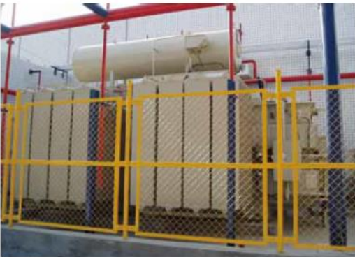
Power Transformer 110kV-100MVA
