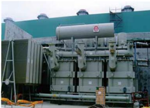
Thermal Power (IPP) Generation Transformer 166kV-386MVA
