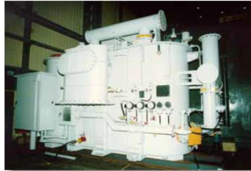
SF 6 Gas-Insulated Transformer 69kV-25MVA
