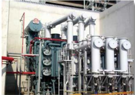
Thermal Power Generation Transformer 345kV-340MVA
