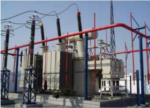
Power Transformer 236kV-150MVA
