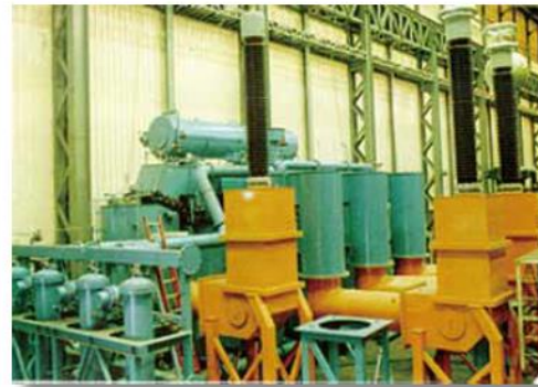
Pumping and Generation Transformer 345kV-300MVA
