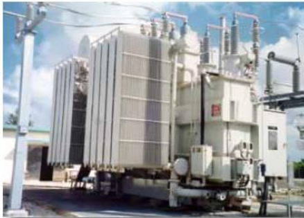
Power Transformer 115kV-112MVA
